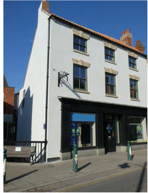
12, Southgate - The old Mark Jarvis Building. A total renovation of this handsome building including new wall rendering and stone window surrounds
